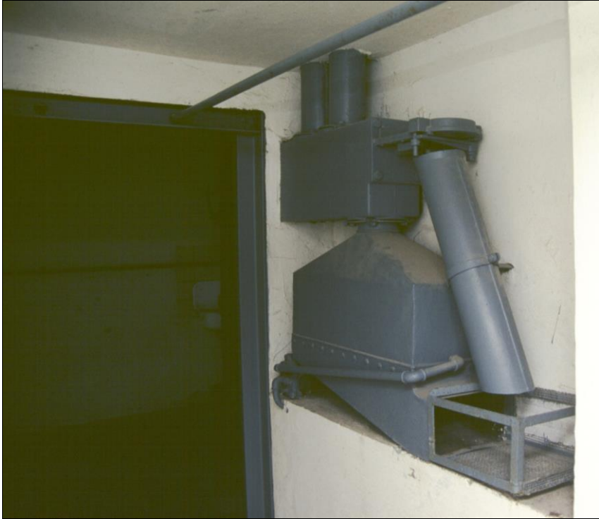
Illustration 23: The inside of one of the four Degesch delousing chambers as it can be seen today in Dachau. At the top, the can opener controlled from the outside. The Zyklon pellets slid through the pipe into a wire-mesh basket at the bottom, through which warm air was conducted by the heater/fan unit (below the can opener).
