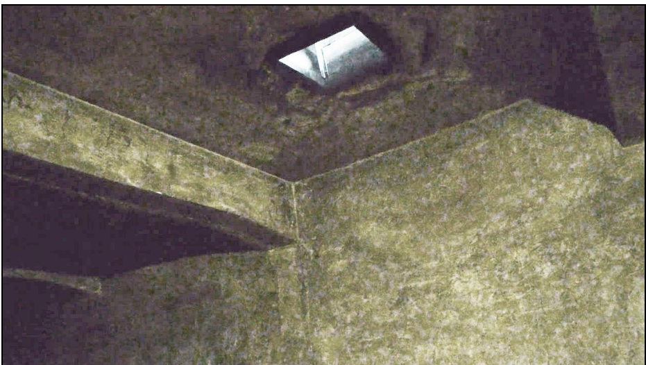
Figure 6: Photograph of hole near original dividing wall and door
